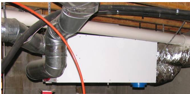
The heat recovery ventilator
